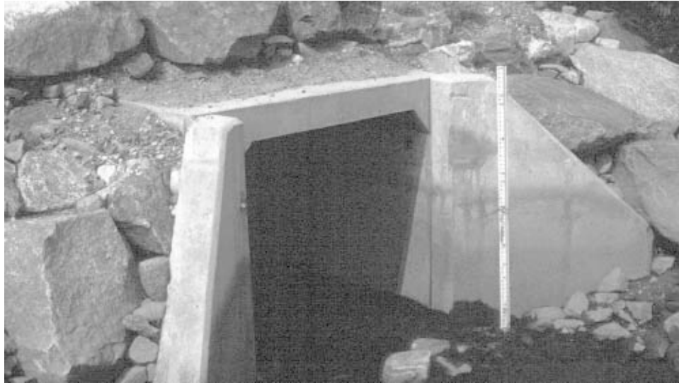
A staff gauge installed on a culvert. Photo: CZM Staff Photo
