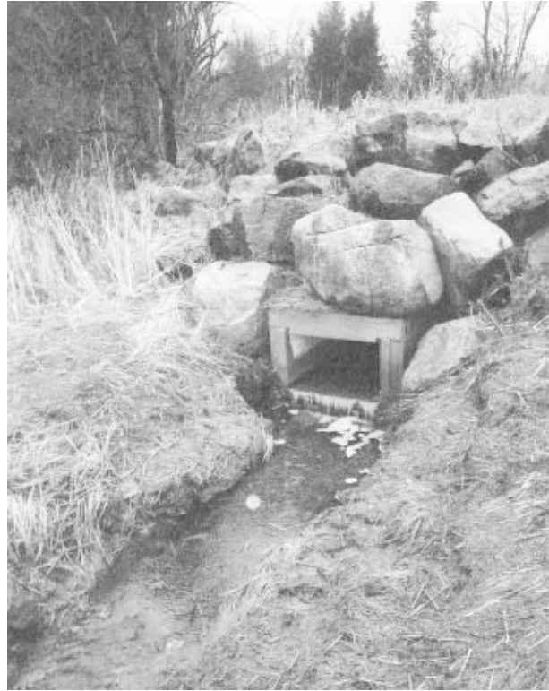
An undersized culvert. Photo: Vivian Kooken
